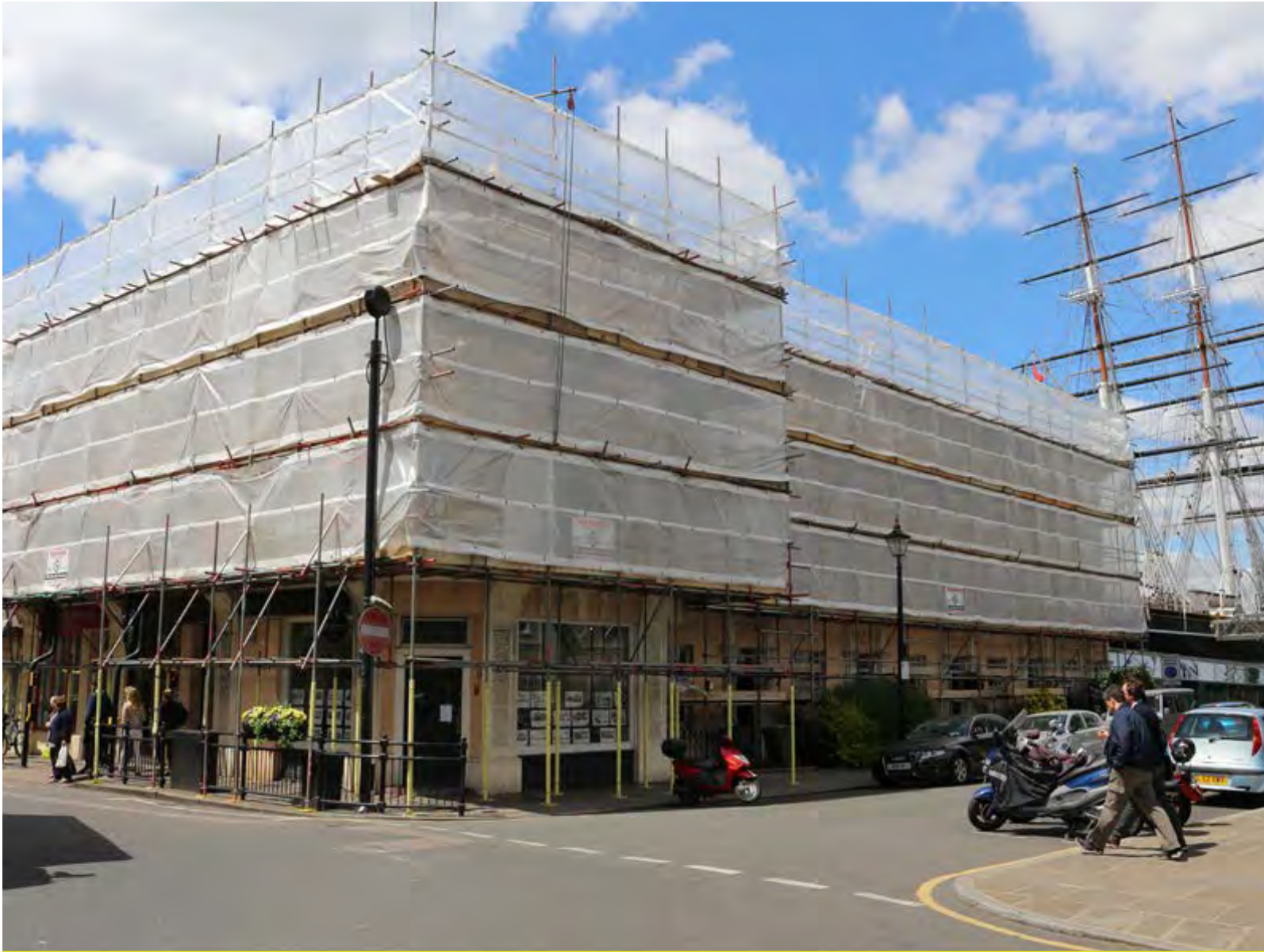
Continuous improvement in Greenwich Town Centre – cleaning and restoration of Greenwich Hospital's property portfolio – 2015
